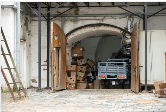
Open loading area with insufficient sealing
